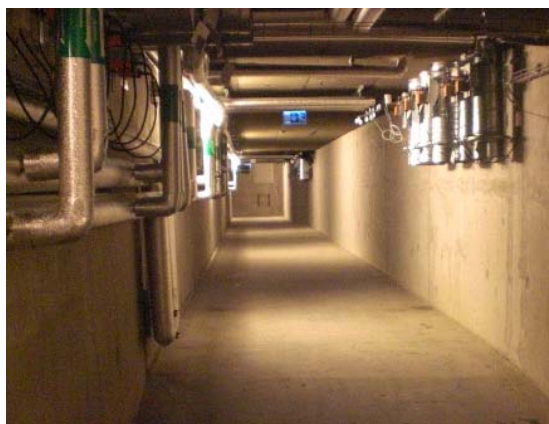
Fig. 6 Supply air dampers and heating valves in supply air ducting. Easily accessible for inspection and adjustment while being out of harms way.
